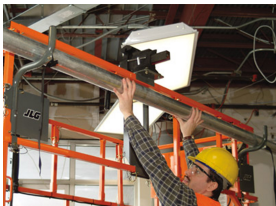
Scissor Lift Pipe Racks
